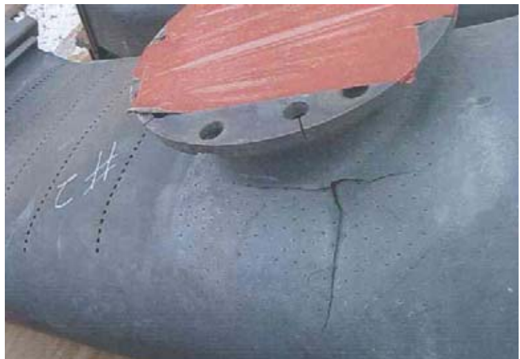
High efficiency with low \text{NO}_x comes at a price. Combustion-driven oscillations have damaged this transition piece from a gas turbine.
